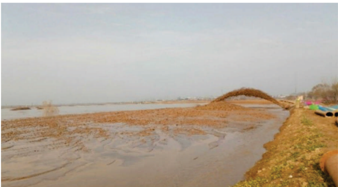
Figure 27: Slurry pump filling
