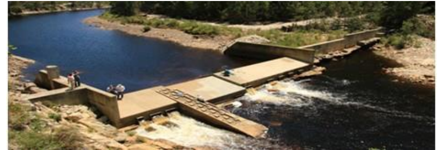
Figure 1. Keurbooms river gauging weir in August 2013 after the 2011 and 2012 flood events, showing damage to the left flank.
