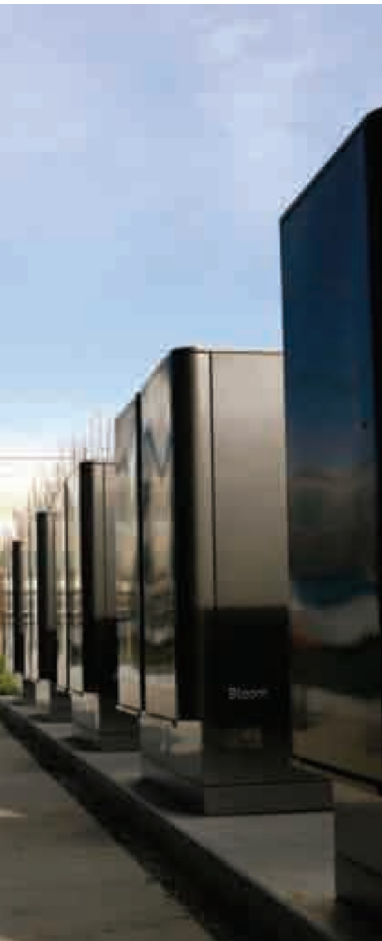
Greener ways to generate electricity, as seen by these Bloom Energy servers in Silicon Valley, are developed through organisations pooling their expertise
